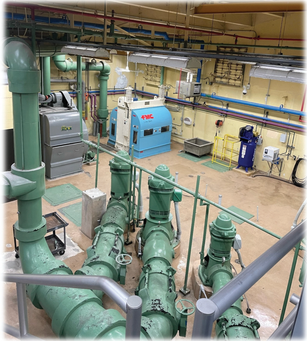
Interior of the Lowlift Pump Station
