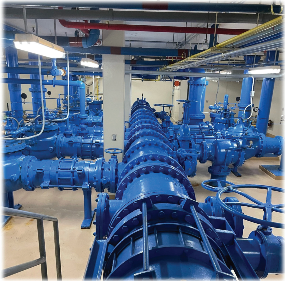
Highlift Discharge Room
