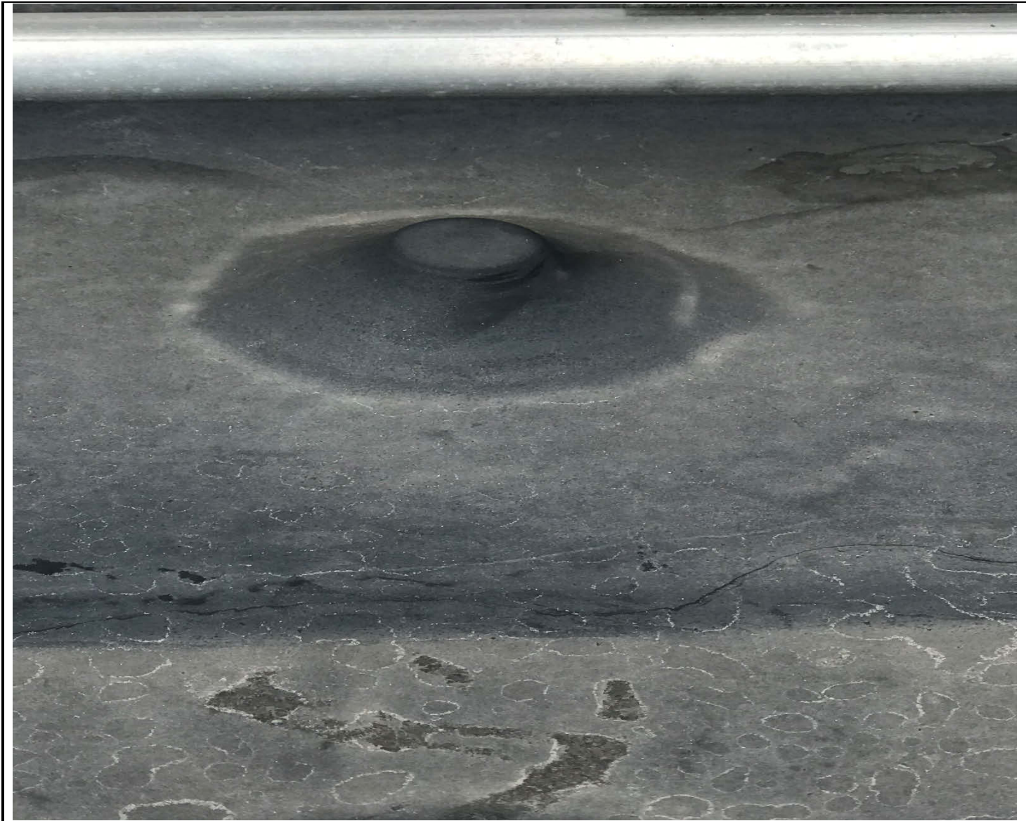
Roof fasteners being pulled out buy ice.
