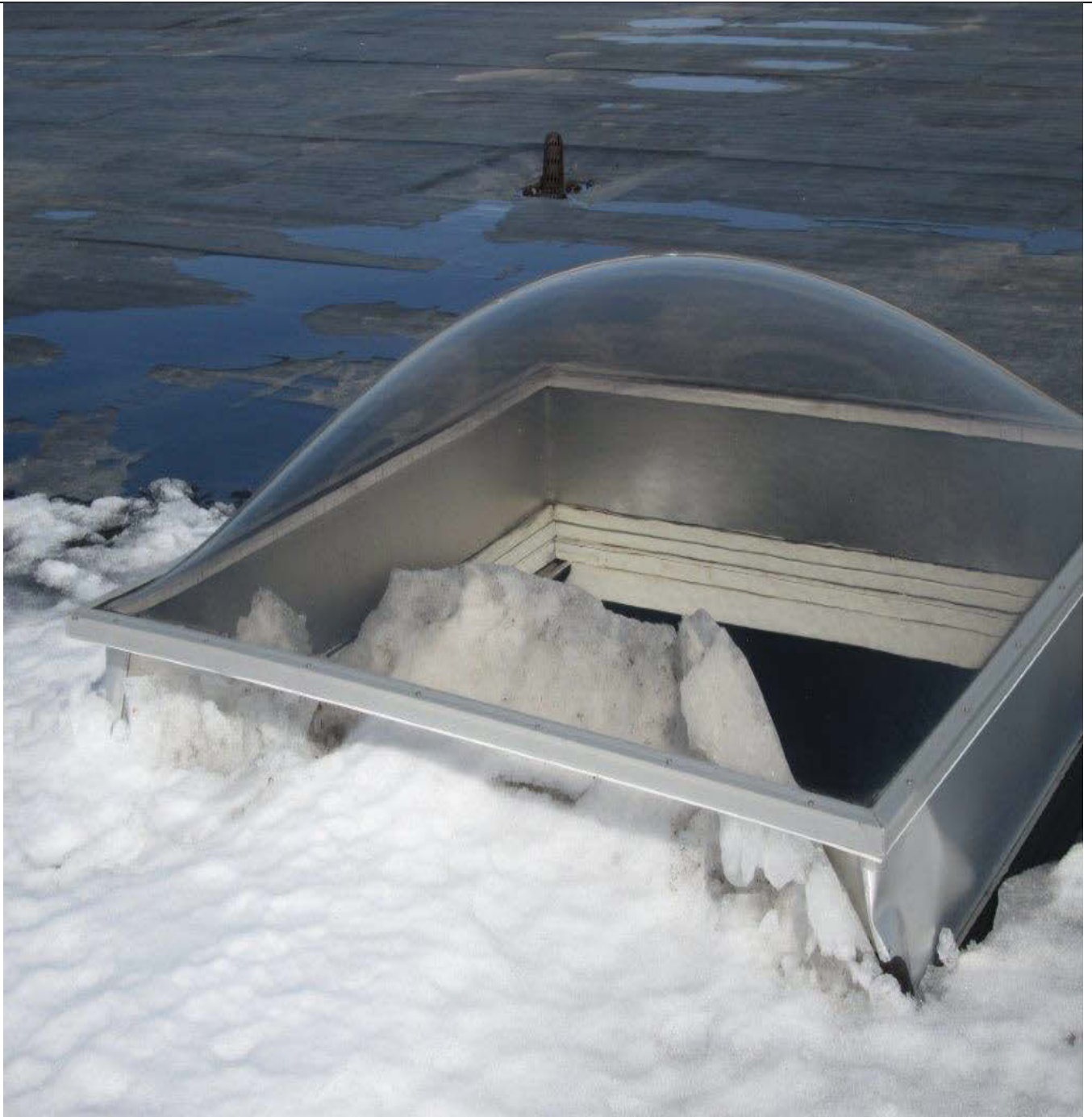
Ice destroyed skylight falling into building.
