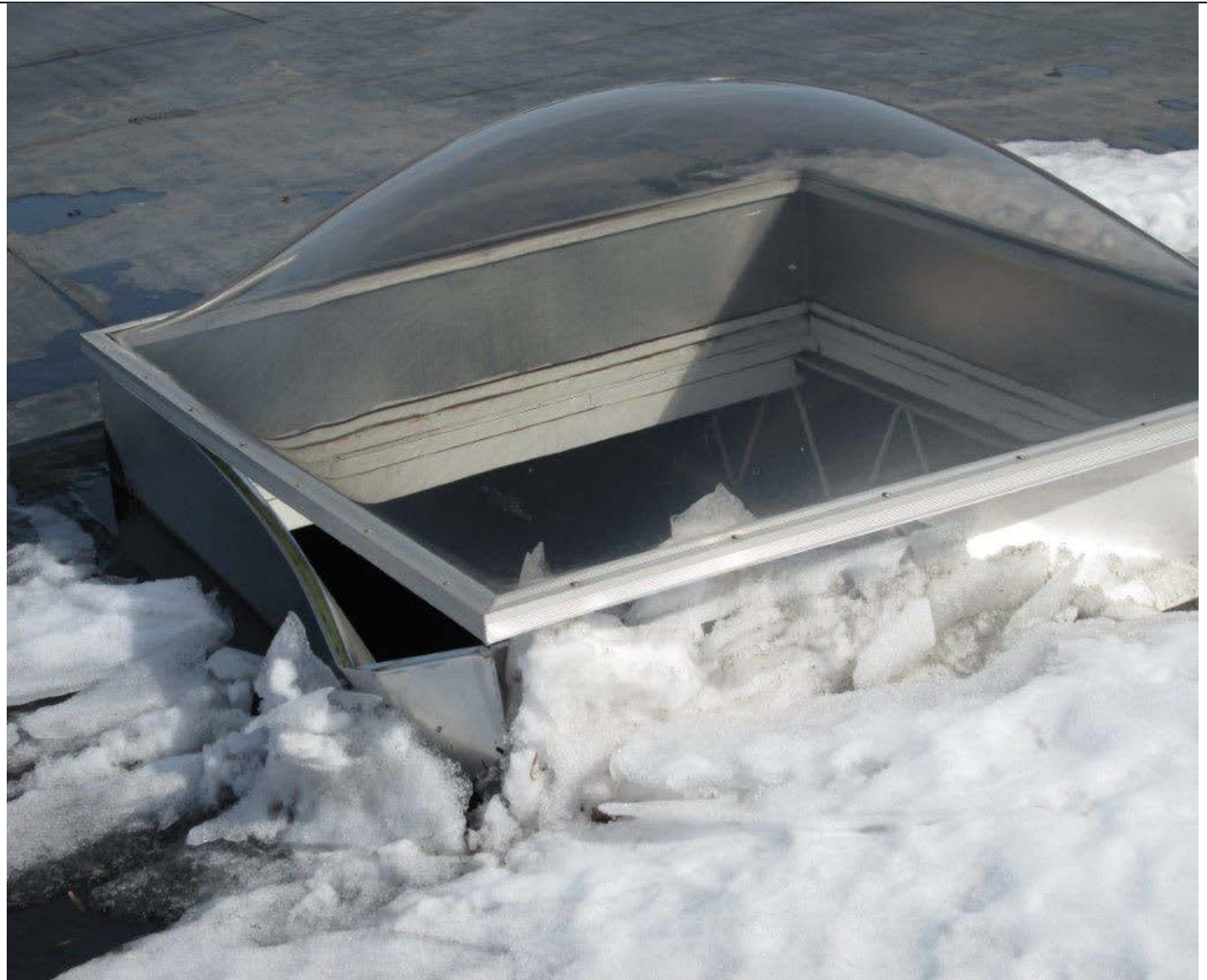
Skylight damage caused by sliding ice.
